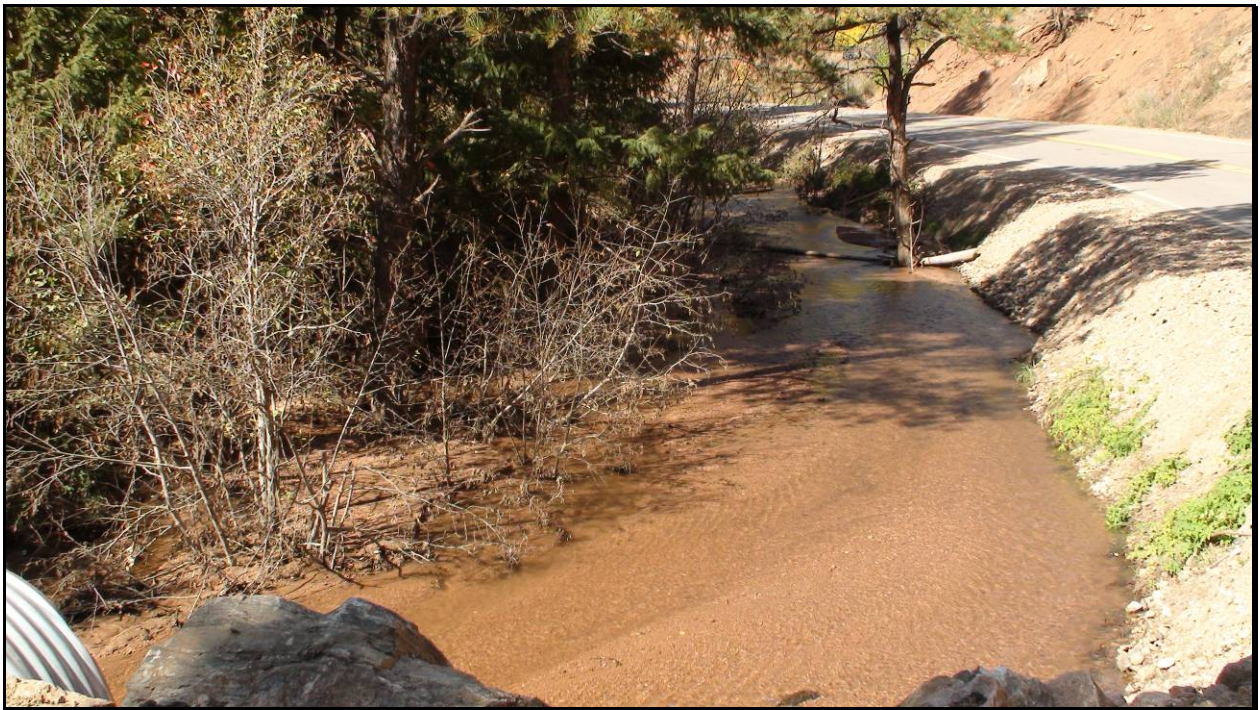
Figure 6. Road fill erosion due to channel encroachment, F4 stream type.
