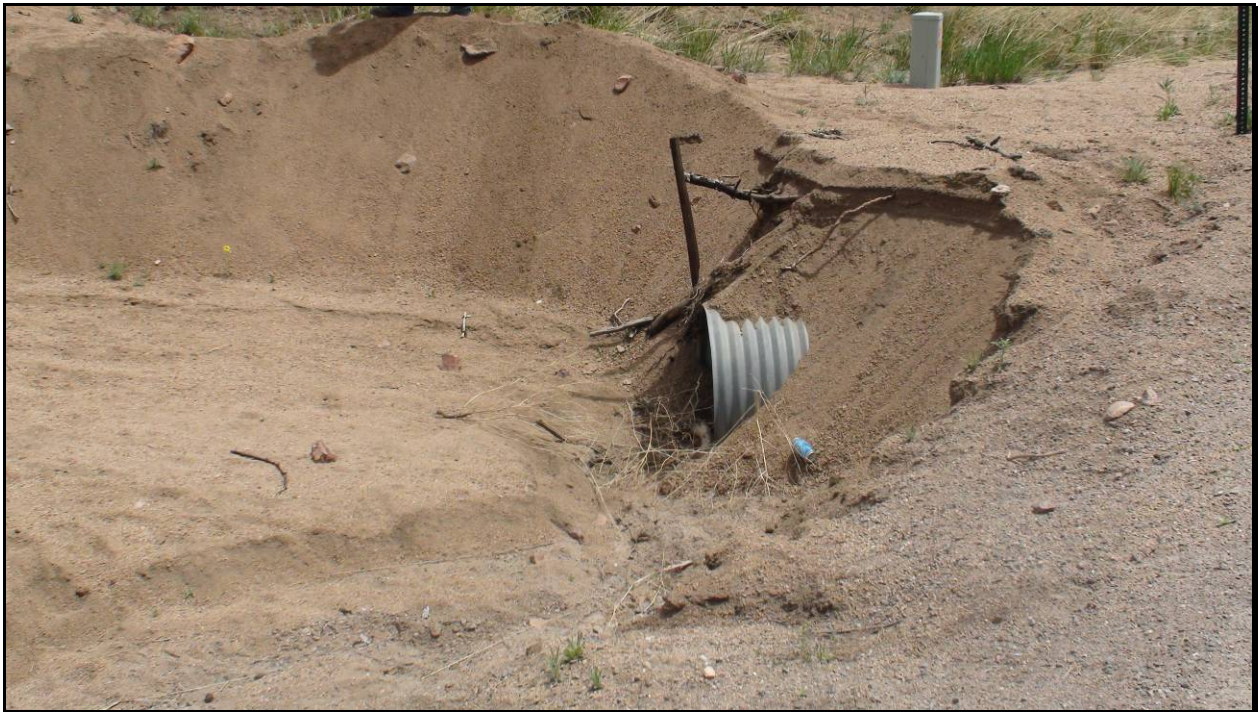
Figure 10. Sediment delivery from poor road drainage.
