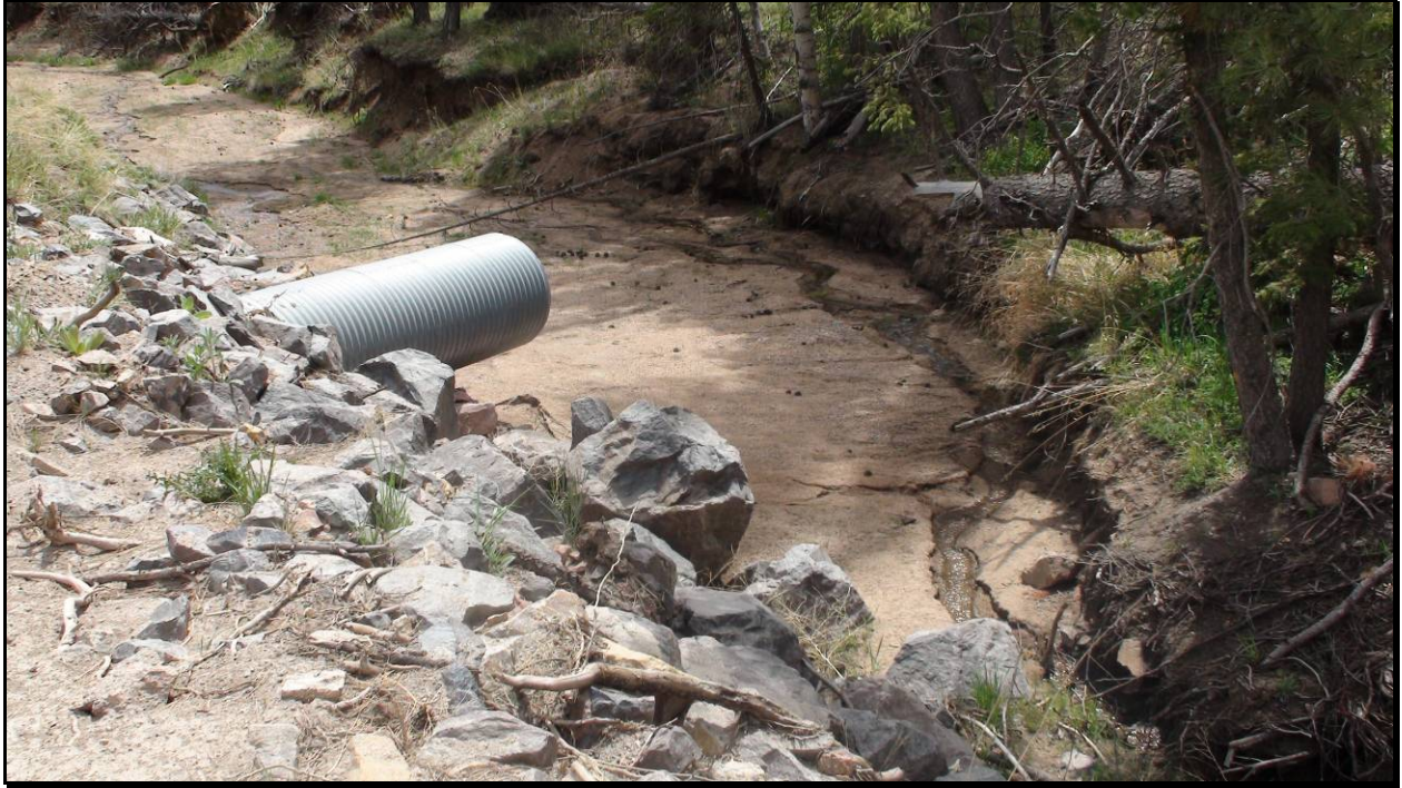
Figure 11. "Shotgun" culvert on tributary to Trail Creek converting a B4 to F4 stream type.
