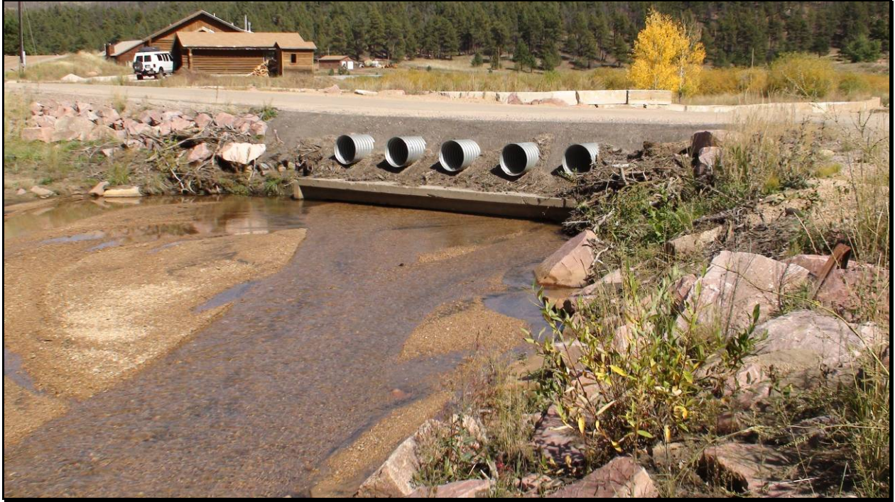
Figure 5. Aggradation due to poor road crossing indicating very high width depth ratio, D4 stream type in Trail Creek.
