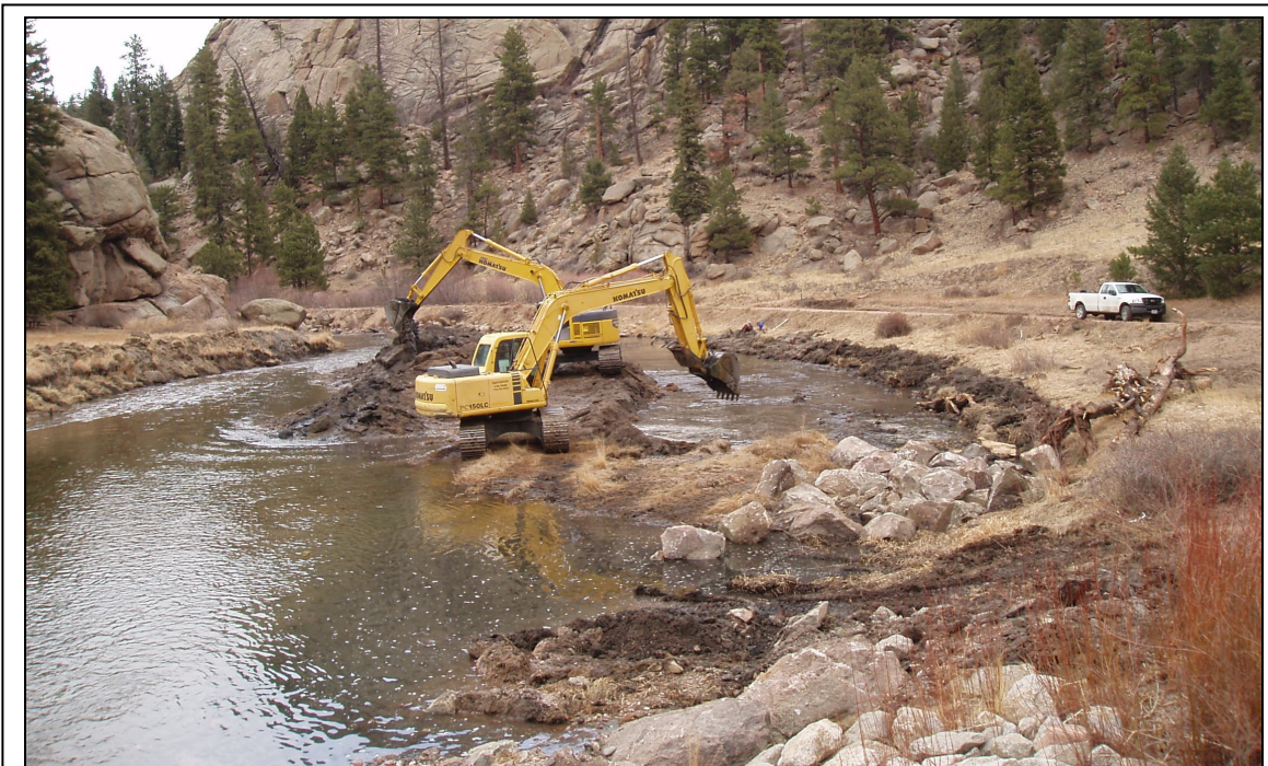
Island removal and river narrowing project. South Platte River - Elevenmile Canyon PG - 2006
